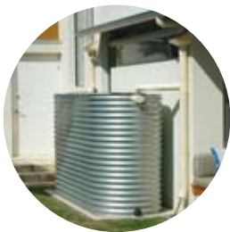
Downspout First Flush Water Diverters and Leaf Eater® filters
